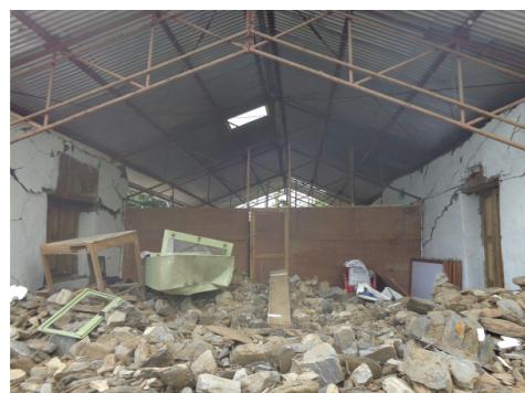
Aftermath of Nepal 2015 Earthquake: Shree Himalaya High (Secondary) School in Sourpanni village
